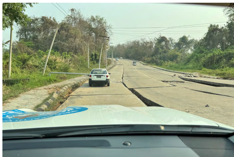
Road damage en route to Nay Pyi Taw, disrupting access for emergency response and humanitarian delivery. ©WCO/Myanmar
