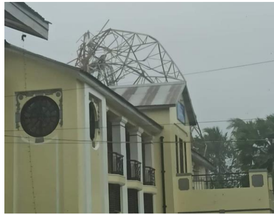
Destroyed telecommunications tower in Sittwe township. Source: Twitter
